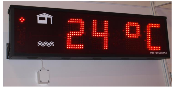
Pool 15 with air temperature sensor
